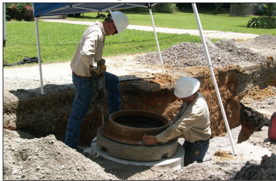
This summer, HU crews replaced 30-year-old sewer mains along Bethel Road in preparation for the new Hartselle High School.
