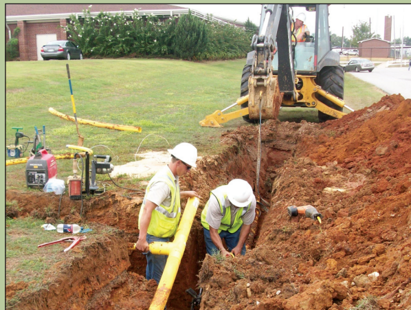
Crews install natural gas pipeline near Danville Middle and Danville High schools.
