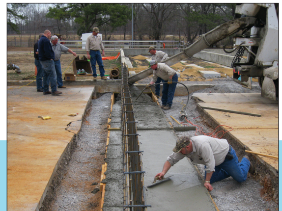
HU crews pour concrete around the drying beds at the wastewater treatment plant.
